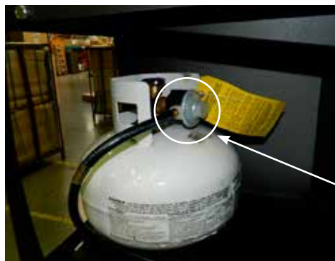
Gas connection @ tank
