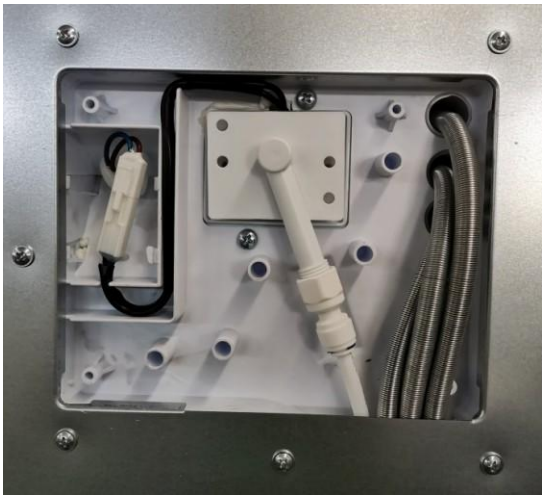
Fill Tube Heaters & Water Lines
