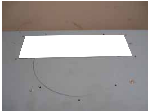
Vertical Ducting (3-1/4"x10" Rectangular)
